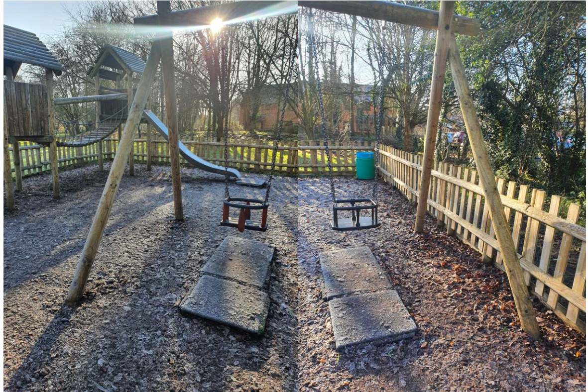
Replace swing frame with new. Keep fixings but install new swings (type tbc)
